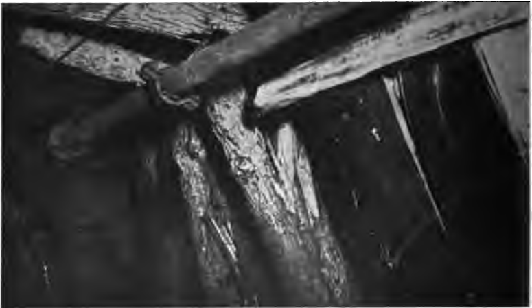
Fig. 12. Broken Timber, Chapin Iron Mine, Oliver Iron Mining Co., Iron Mountain, Mich.
